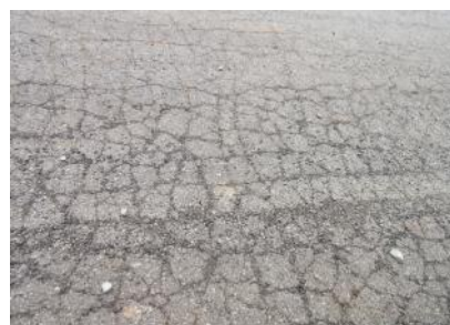
Extensive damage found along Talon Ridge Ct.
