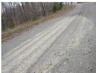
Extensive damage found along Talon Ridge Ct.
