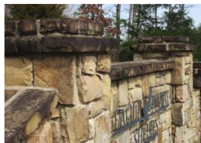
Stone will need to be cleaned.
